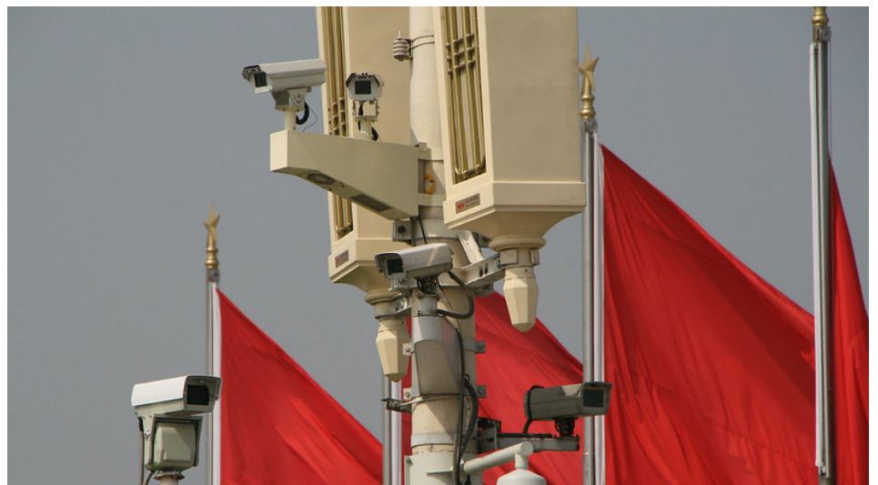
Surveillance cameras installed in Tiananmen Square, Beijing (Source: Jack Hynes/Flickr)
