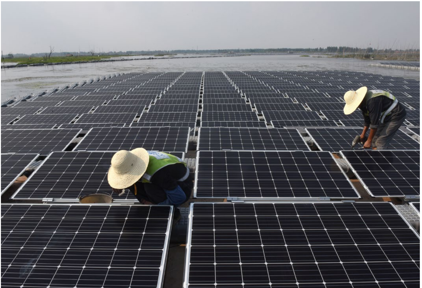
Chinese workers install panels at the Huainan solar farm in Anhui province. Constructed on the site of a former coal mine and comprising over 160,000 solar modules, the array is one of the world's largest floating photovoltaic solar plants and has capacity to power more than 15,000 homes (2017).
